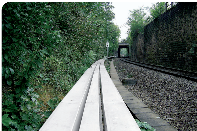
Three parallel cable ducts on one support
